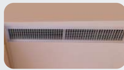
Front air flow, back air intake
